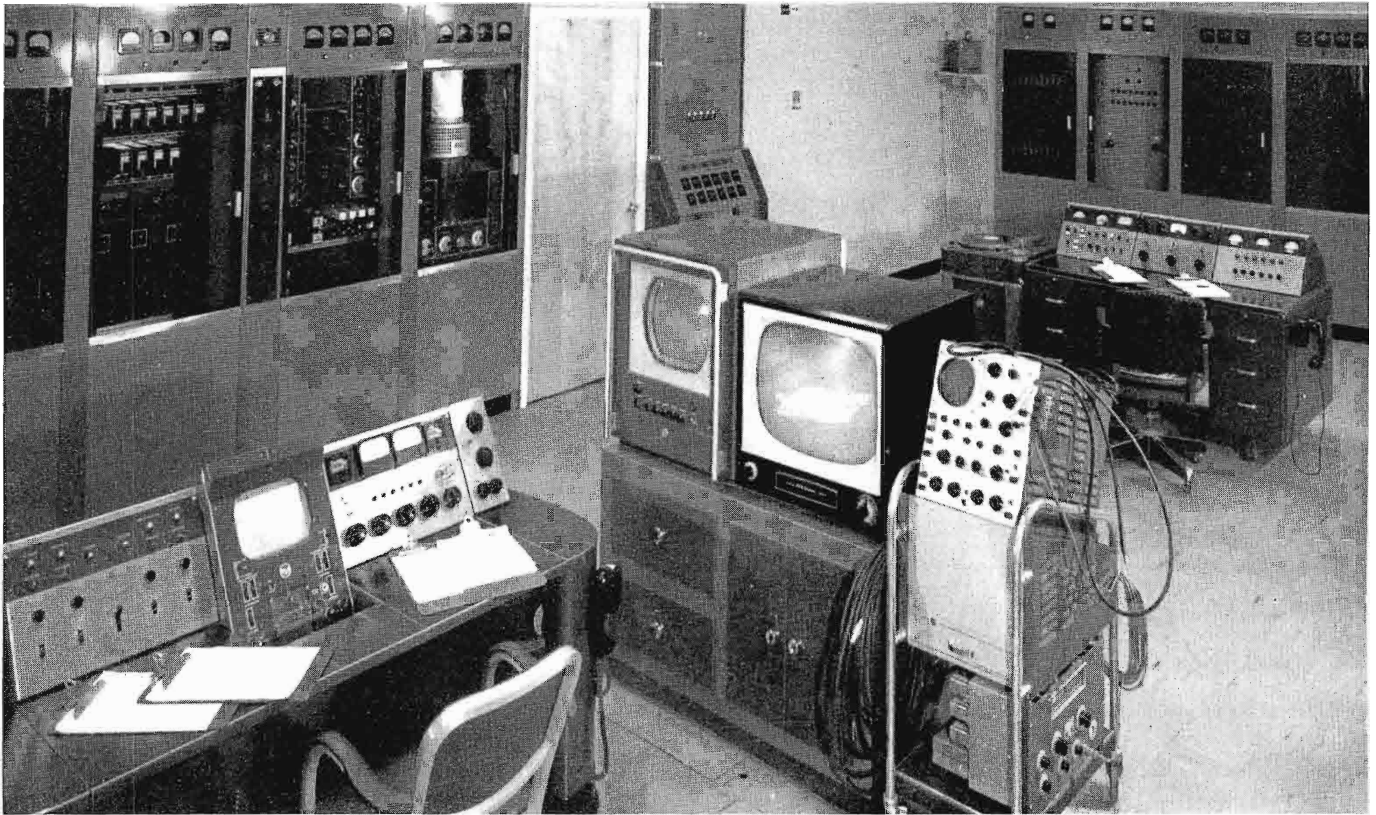
FIG. 3. View of transmitter room. TV console and portion of TV transmitter at left. AM console and portion of BTA-5H AM transmitter at upper right.
