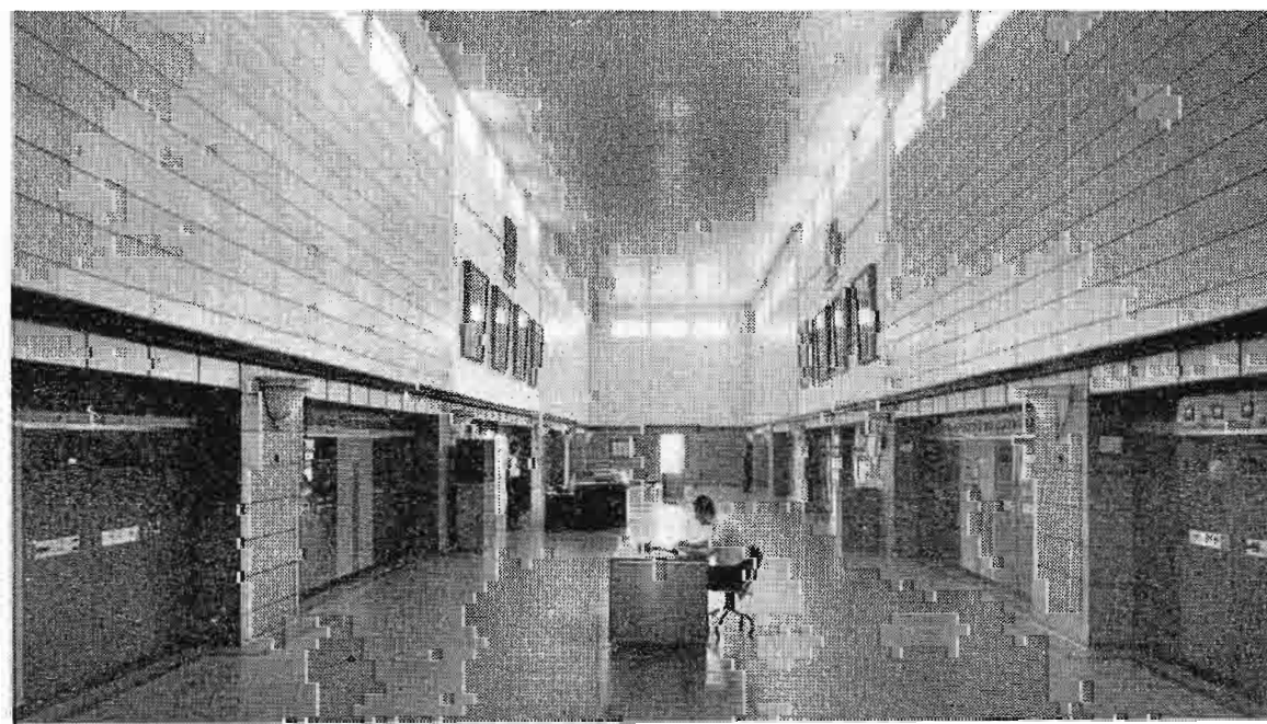
FIG. 12. At the transmitter center in Portugal 13 broadcast transmitters are used to beam programs to target countries. Shown here is the main transmitter hall housing eight RCA 50-kw transmitters.
