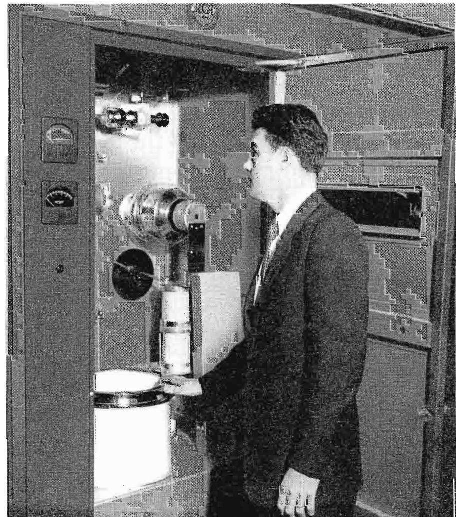
FIG. 5. Inspecting the right hand PA cabinet is William Sadler, KSTP's Chief Engineer. Note the generous over-size plate tuning capacitor. Vacuum capacitors are used in all stages to guarantee maximum dependability.
