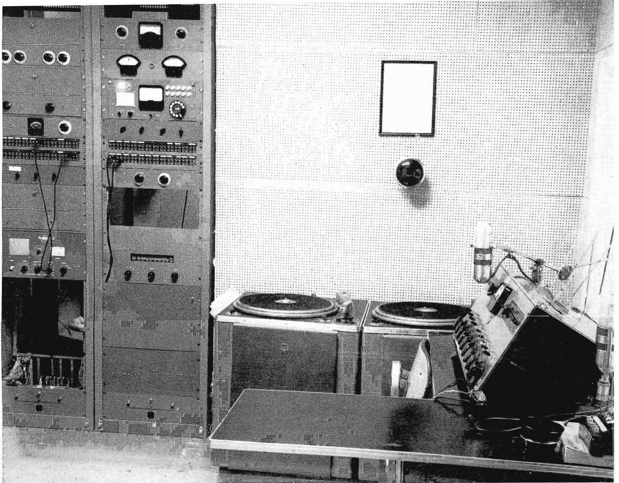
FIG. 3. Complete equipment facilities in Control Room A include a BC-2B Consolette, two BQ-2A Turntables and two equipment racks.
