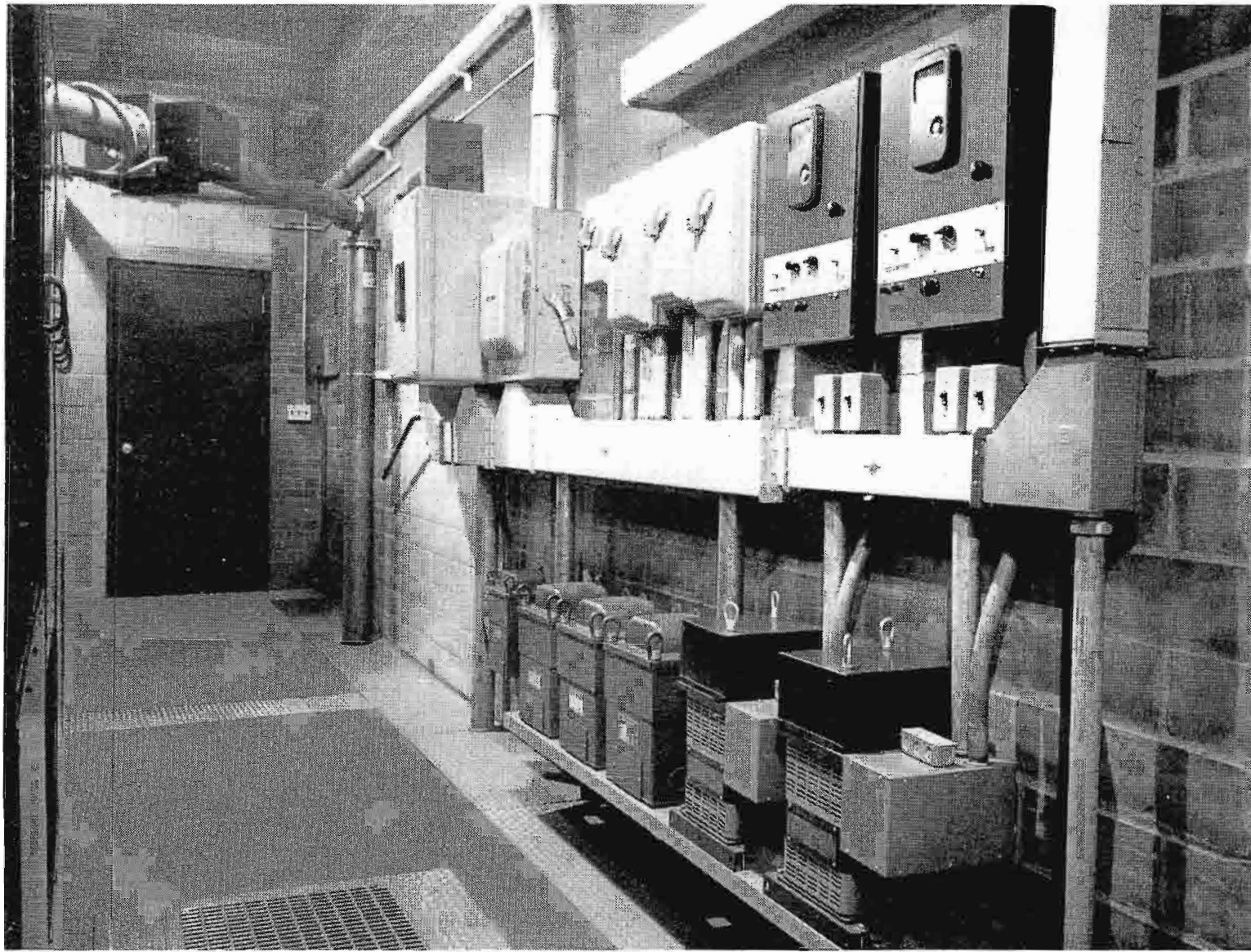
FIG. 6. KSTP chose to modify the typical arrangement of the wall-mounted switch gear—frankly, we feel that they have improved the arrangement. In the typical layout, the distribution transformers are mounted at the upper right at eye level—KSTP has installed all heavy components at floor level which eliminates the necessity for reinforcing the tile wall. Starting at the upper left, the top of the main line 400 amp/600 volt disconnect switch can be seen. This is the only piece of switch gear which must be supplied by the customer. Next in line is the plate breaker, a Delta-Wye switch, and the low-power, intermediate and distribution breakers. The two units to the right are the contact making voltmeters for the two voltage regulators at floor level. The three transformers to the left are the 460/230 volt distribution transformers which supply regulated voltage to the filament control circuits. The door to the rear gives access to the transformer vault and is interlocked for personnel protection. The clear layout is typical of the sound engineering practices used at KSTP.
