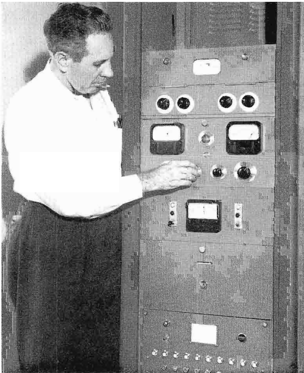
FIG. 9. W. D. Cousar, who maintains all equipment at WHER, checks readings at switching unit of remote control system in transmitter building.
